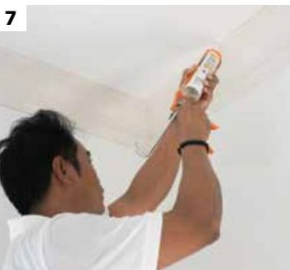
7 For any pits that exist between moulding, it's better to fill with putty or A,B glue after installation
