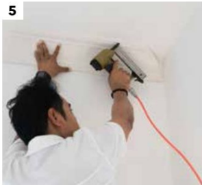
5 Fix the moulding on the marked wall surface and ceiling with steel nail, and then fill the nail beads with stuccowork
